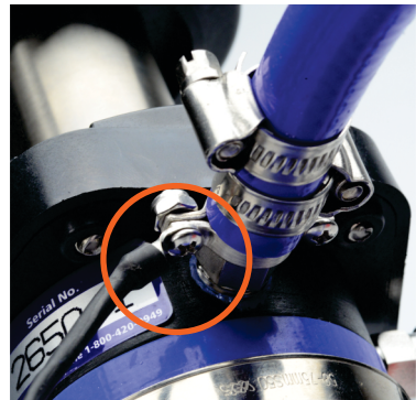
Sensor Mounted On Shaft Seal Injection Fitting
